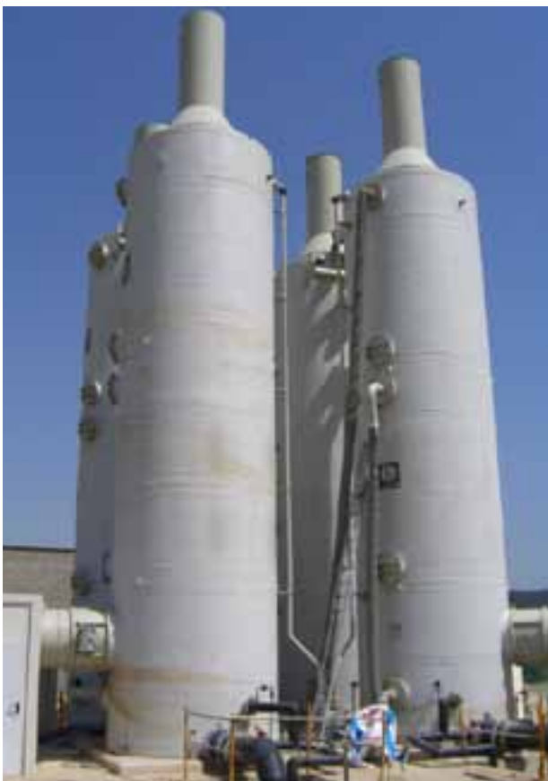
Degassing (stripping) of aquifer water
