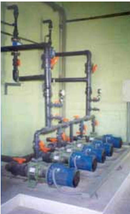
Truck discharge pumps
