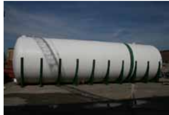
Brine, softened water, CIP process tank and reagent storage tanks
