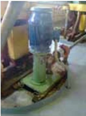
Manhole and wash water collection pumps
