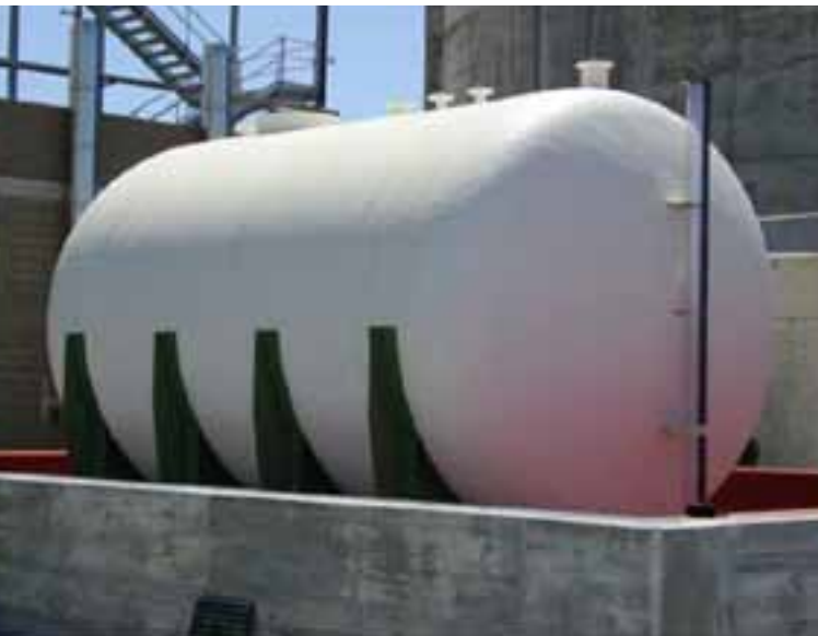
Reagent storage tanks
