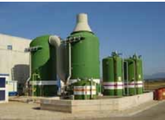
Deodourisation at urban WWTP with 2 chemical treatment stages ( H_2SO_4 / NaOCl + NaOH ) for Q = 50.000 \text{ m}^3/\text{h}
