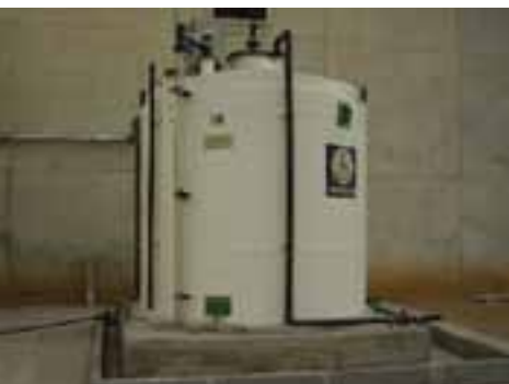
Double-walled reagent storage tanks
