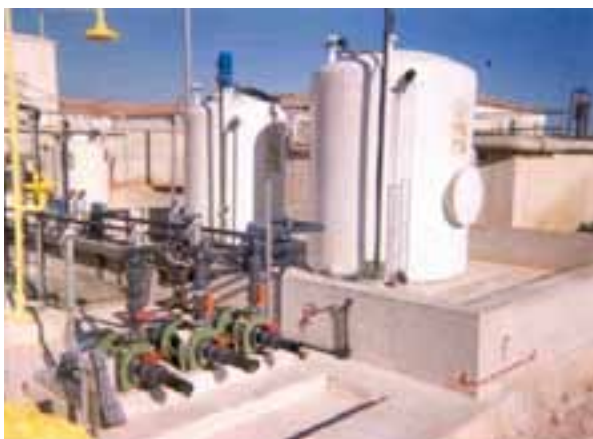
Truck discharge pumps
