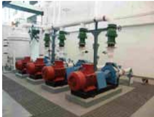
Pumps for membrane cleaning
