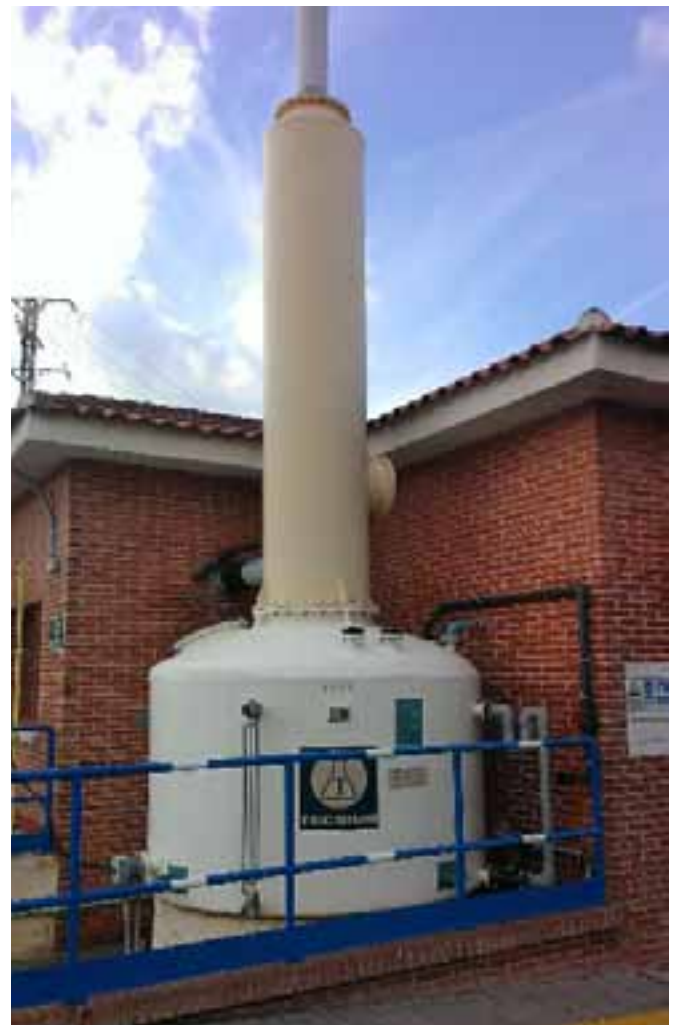
Chlorine leak emergency installation
