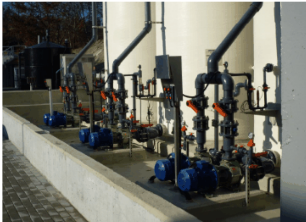
Reagent transfer pumps and transfer to consumption points
